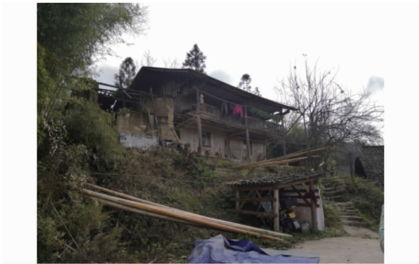
图 2 失修的特色建筑 Fig. 2 Dilapidated characteristic architecture
